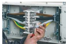
Conductor ends need to have the oxide layer carefully scraped clean.
