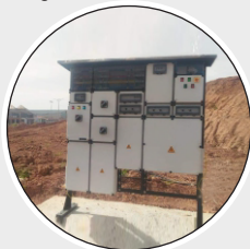
Power Distribution Panels
