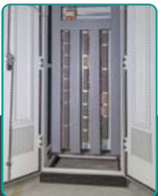
Cable Marshalling Panels
