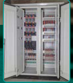
Power Distribution Boards
