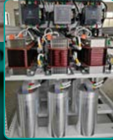
Power Factor Improvement Panels
