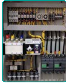
Auto Transfer Switch Panels
